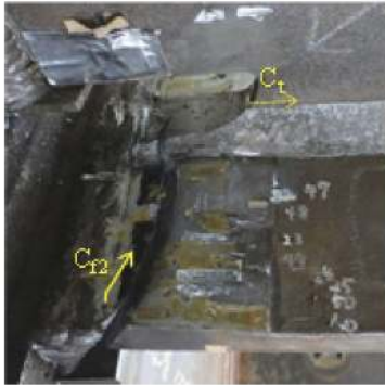
(a) No. 1 : Flange fracture at beam-end weld
