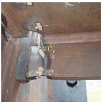
(c) No. 5 : Flange fracture at beam-end weld scallop
